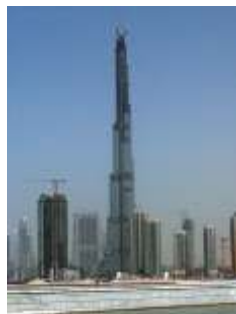
The Burj Dubai (Dubai Tower) construction site workers are using ISGUS Perfect Time Recorders for their presence recording.
